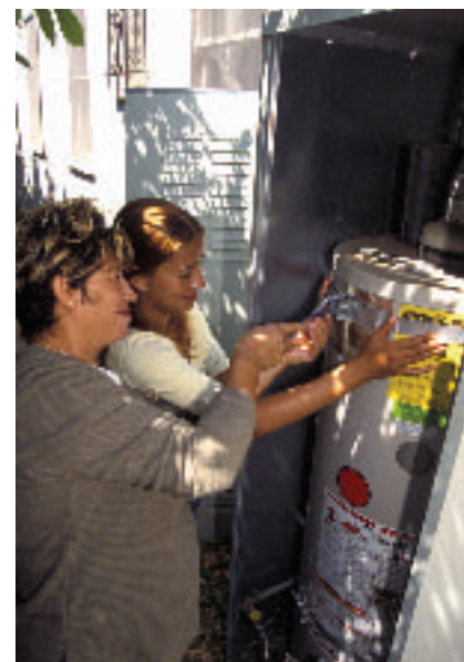
Figure 22 Sturdy metal straps on this gas water heater help reduce the danger of fires from broken gas lines during an earthquake.
