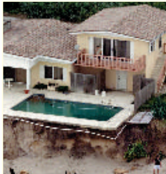
This beach house will collapse as its underpinnings are eroded.
